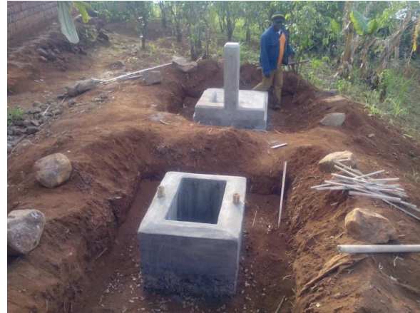
Standpipe and meter chamber at Bongeh/Shuashua
